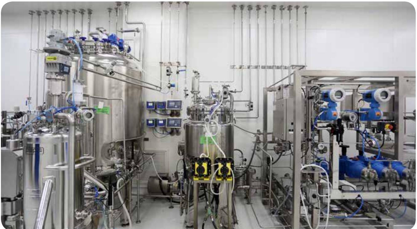
Production complexity and recipe variety compounded the challenge, requiring the development of tailor-made process applications capable of supporting more than 300 phases and 70 recipes
